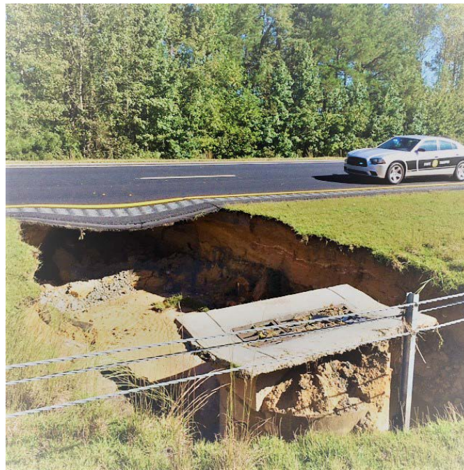
FIGURE 5.12: SINKHOLE IN NORTH CAROLINA
