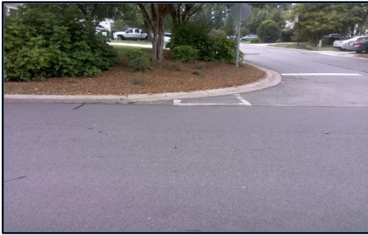
Corner 1 No Ramp (1z)
