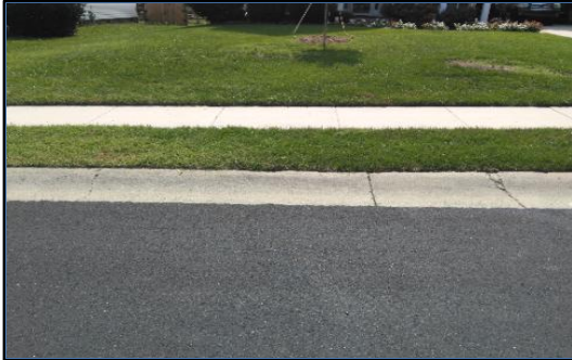
Corner 3 No Ramp (3z)
