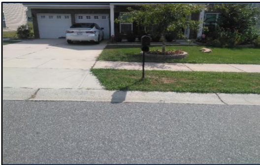
Corner 3 No Ramp (3z)
