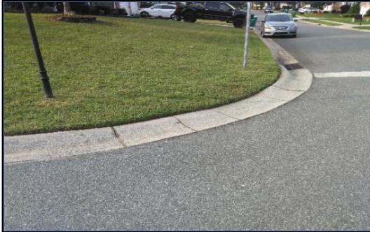
Corner 3 No Ramp (3z)
