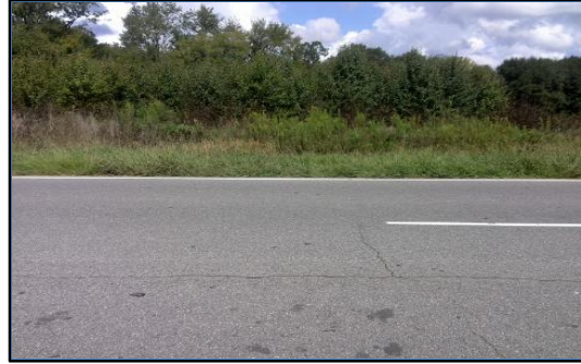
Corner 2 No Ramp (2z)
