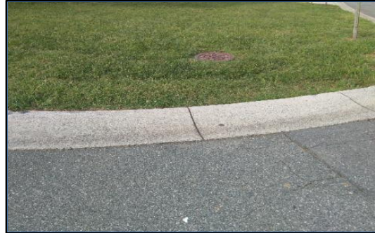
Corner 4 No Ramp (4z)
