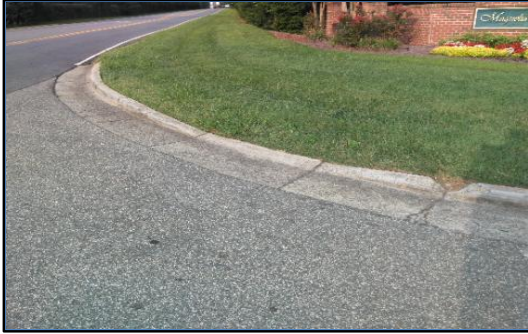
Corner 1 No Ramp (1z)
