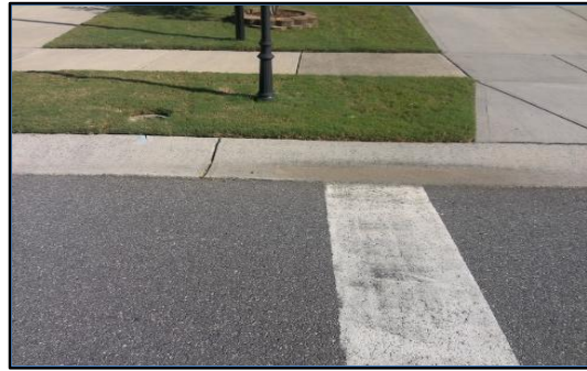
Corner 2 No Ramp (2z)
