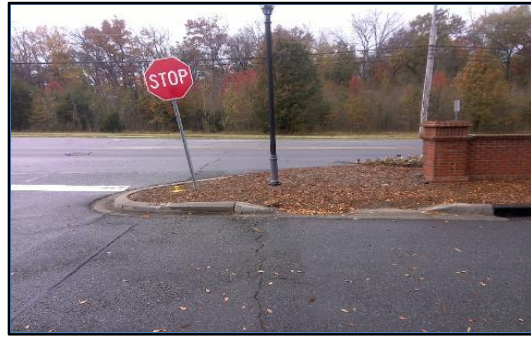
Corner 1 No Ramp (1z)
