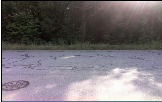
Corner 3 No Ramp (3z)
