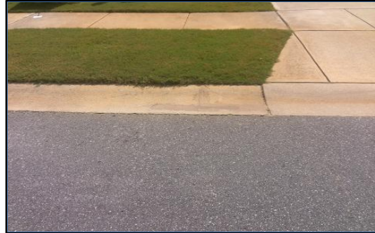
Corner 3 No Ramp (3z)
