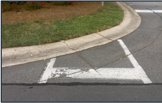
Corner 1 No Ramp (1z)
