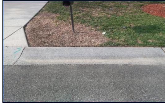
Corner 4 No Ramp (4z)
