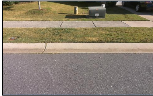
Corner 2 No Ramp (2z)
