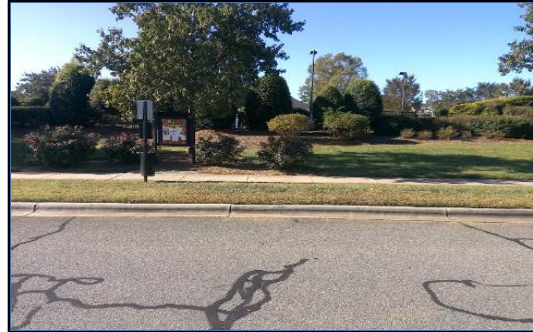
Corner 4 No Ramp (4z)
