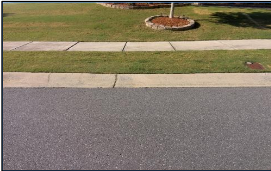
Corner 3 No Ramp (3z)
