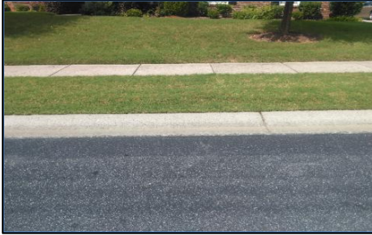
Corner 1 No Ramp (1z)
