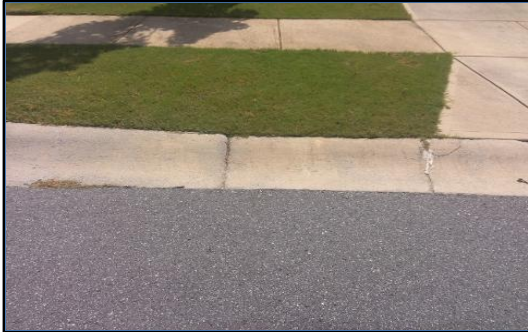
Corner 2 No Ramp (2z)
