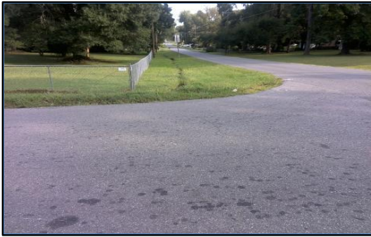
Corner 1 No Ramp (1z)
