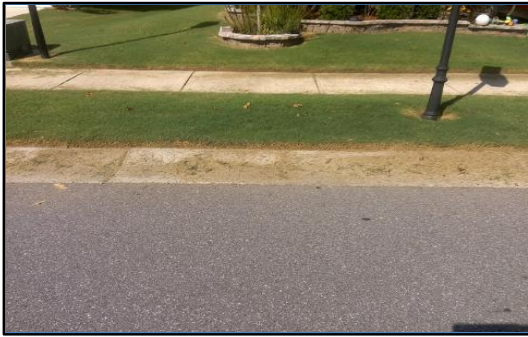
Corner 1 No Ramp (1z)
