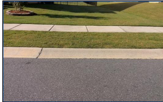
Corner 4 No Ramp (4z)
