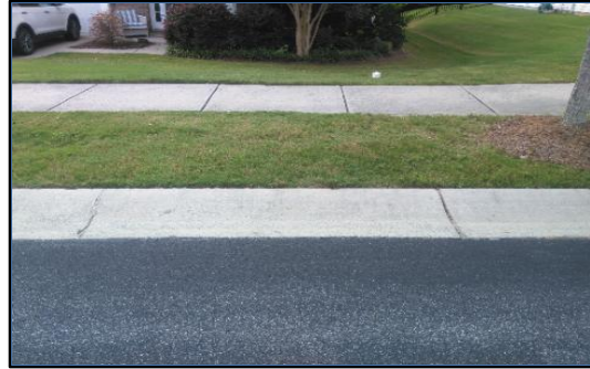
Corner 4 No Ramp (4z)
