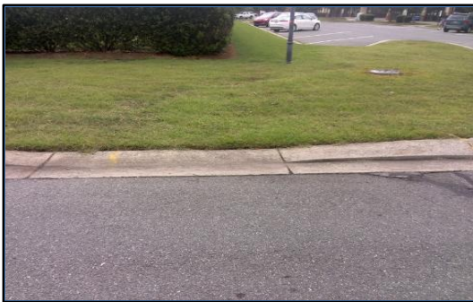
Corner 4 No Ramp (4z)
