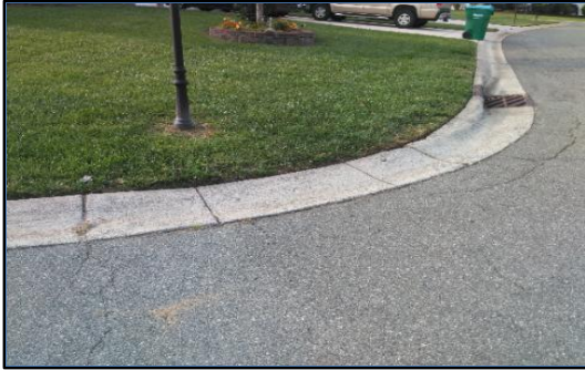
Corner 3 No Ramp (3z)
