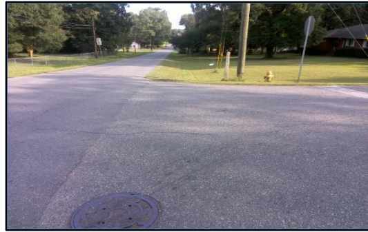
Corner 2 No Ramp (2z)
