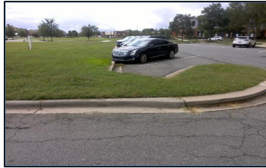
Corner 3 No Ramp (3z)
