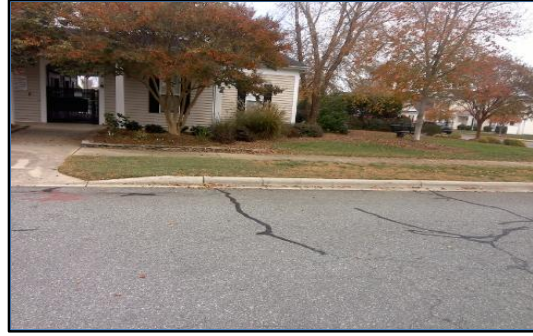
Corner 2 No Ramp (2z)
