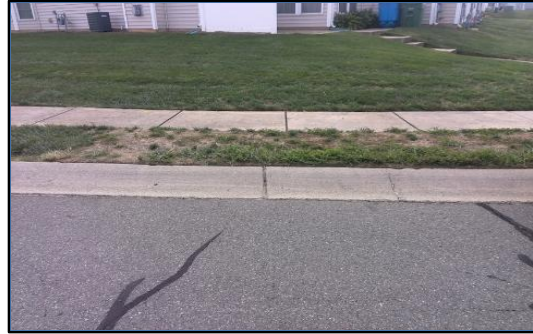
Corner 4 No Ramp (4z)
