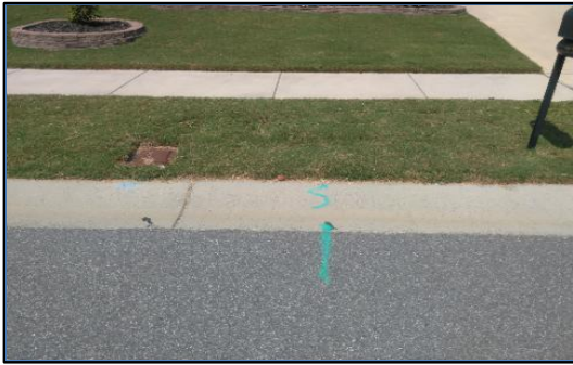
Corner 1 No Ramp (1z)
