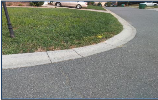
Corner 1 No Ramp (1z)
