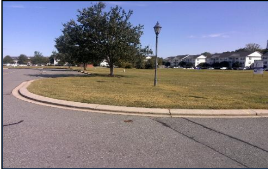
Corner 2 No Ramp (2z)
