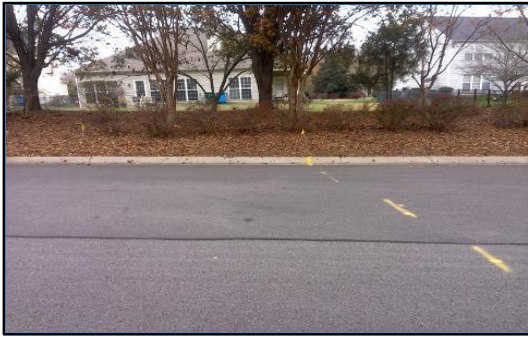
Corner 1 No Ramp (1z)
