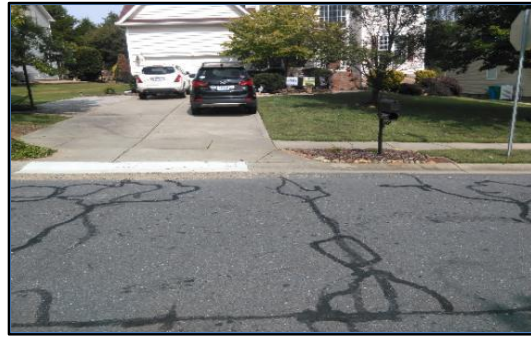
Corner 2 No Ramp (2z)
