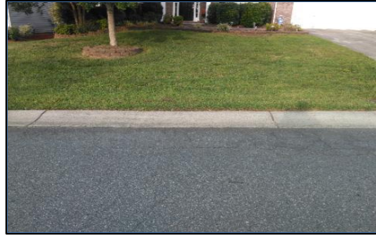
Corner 4 No Ramp (4z)
