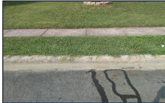
Corner 4 No Ramp (4z)
