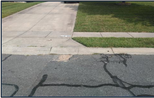
Corner 1 No Ramp (1z)
