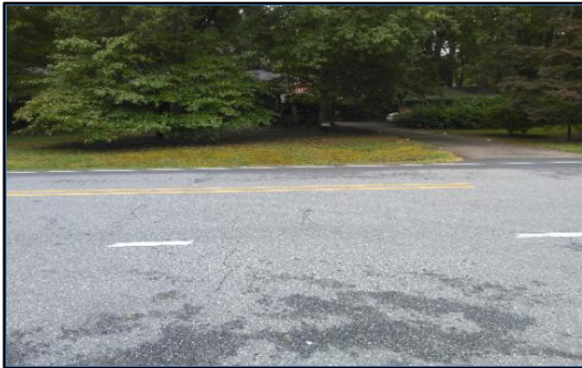
Corner 3 No Ramp (3z)
