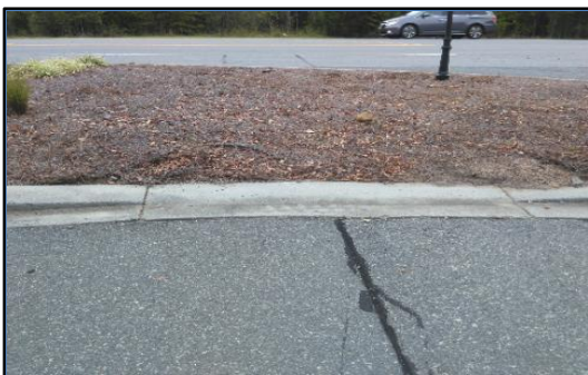
Corner 4 No Ramp (4z)
