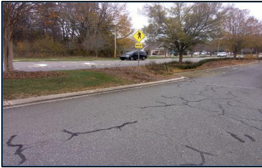
Corner 1 No Ramp (1z)
