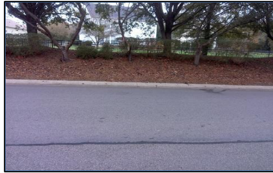
Corner 2 No Ramp (2z)
