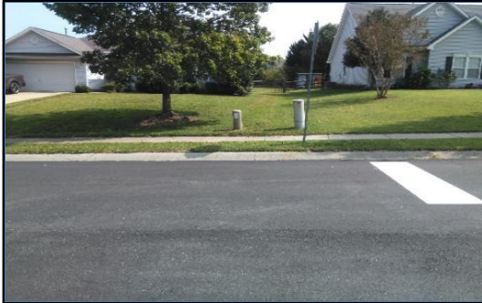
Corner 3 No Ramp (3z)
