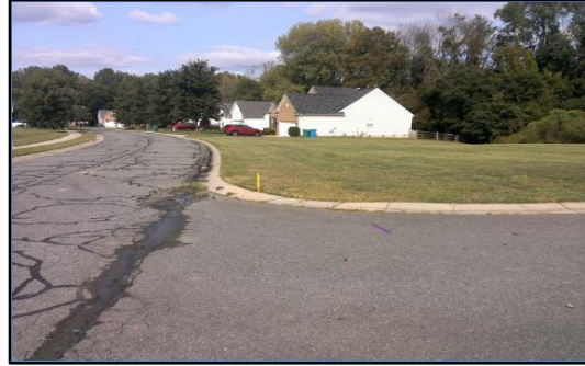
Corner 3 No Ramp (3z)
