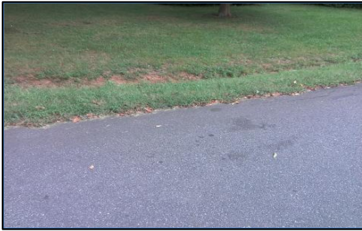
Corner 1 No Ramp (1z)
