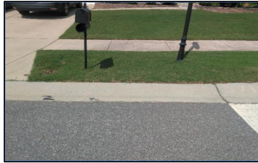
Corner 2 No Ramp (2z)
