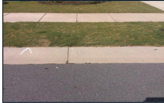
Corner 4 No Ramp (4z)
