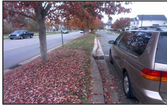
Corner 1 No Ramp (1z)
