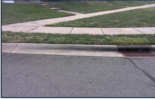
Corner 1 No Ramp (1z)
