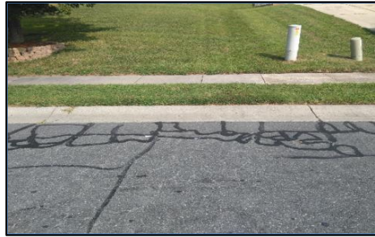
Corner 2 No Ramp (2z)
