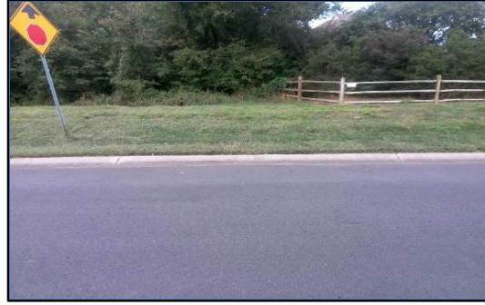
Corner 2 No Ramp (2z)
