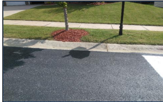
Corner 4 No Ramp (4z)
