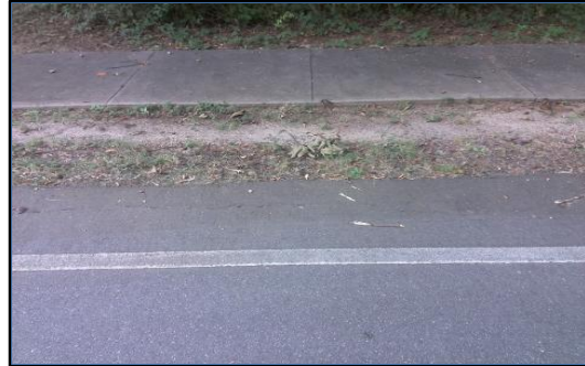
Corner 4 No Ramp (4z)
