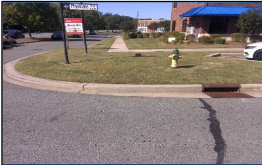
Corner 2 No Ramp (2z)
