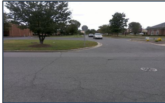
Corner 4 No Ramp (4z)
