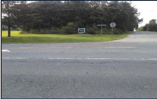
Corner 3 No Ramp (3z)
