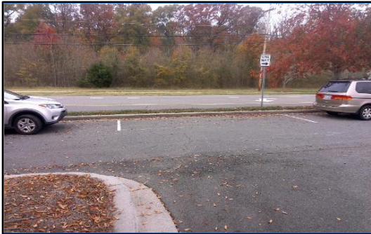
Corner 4 No Ramp (4z)
