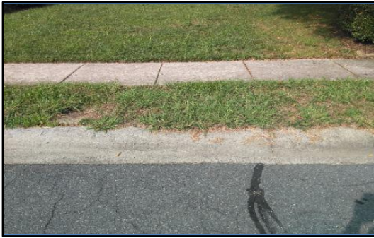
Corner 1 No Ramp (1z)
