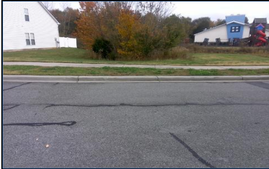
Corner 3 No Ramp (3z)
