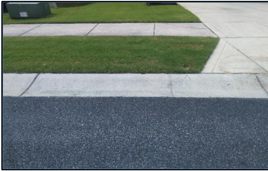
Corner 1 No Ramp (1z)
