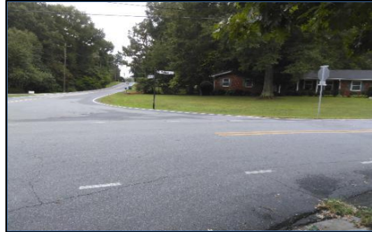
Corner 4 No Ramp (4z)
