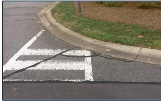
Corner 2 No Ramp (2z)
