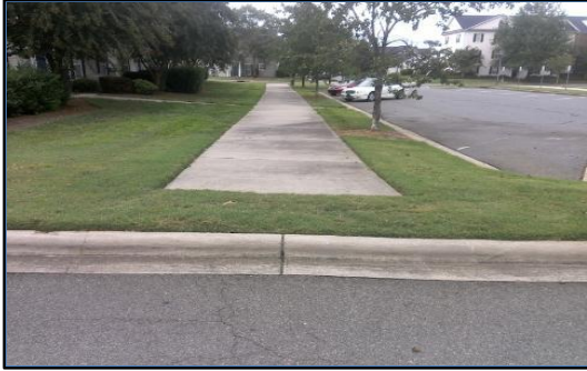
Corner 1 No Ramp (1z)
