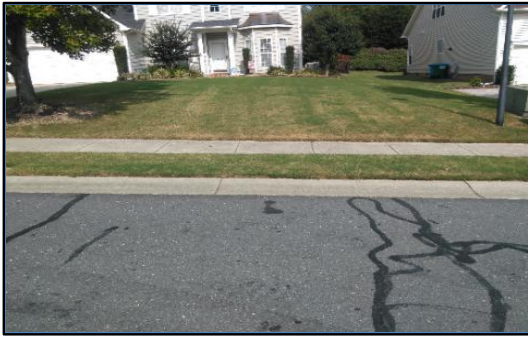
Corner 1 No Ramp (1z)
