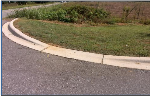
Corner 3 No Ramp (3z)
