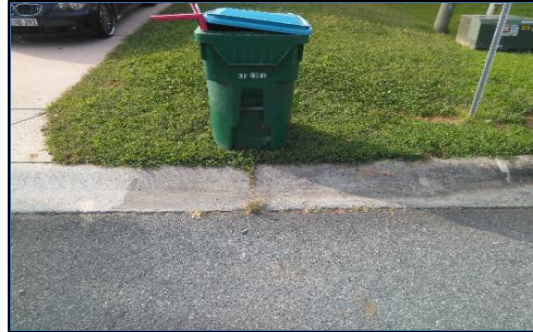
Corner 4 No Ramp (4z)
