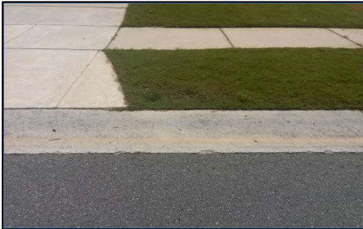
Corner 3 No Ramp (3z)
