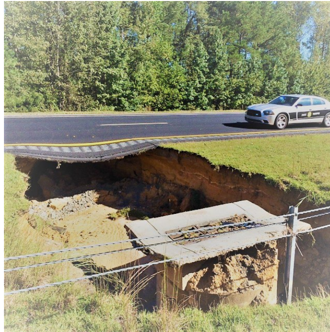
FIGURE 5.13: SINKHOLE IN NORTH CAROLINA
